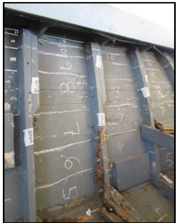
Figure 20. Image showing the port planking above the chine, with the beginning of the eleventh strake in line with the tops of the second futtock indicating the original height of the hull (Photograph by Jeremy Borrelli, 2013).
