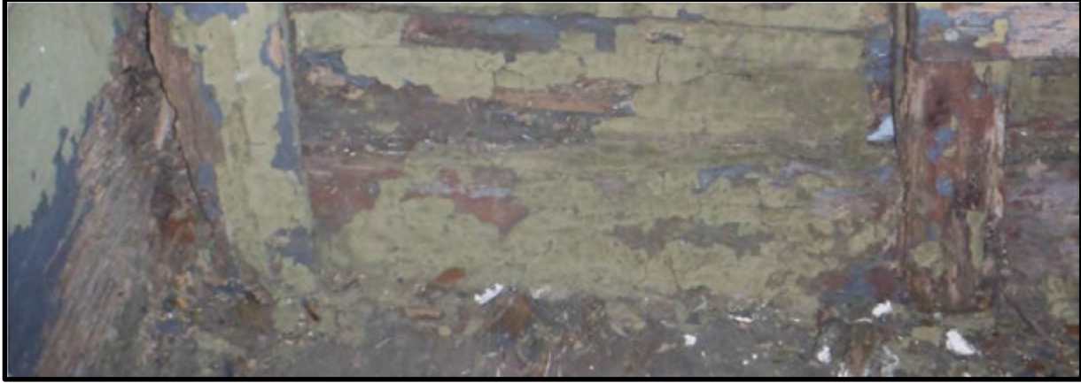
Figure 45. Deteriorated condition of aft port stringer. (Photo by Ryan Bradley, 2013).
