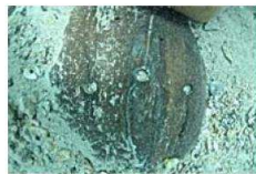
17-IMG_187-N timber fastener hole
