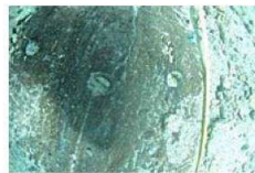
18-IMG_188-N timber fastener hole
