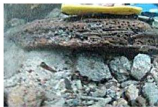
16-IMG_186-S timber thickness
